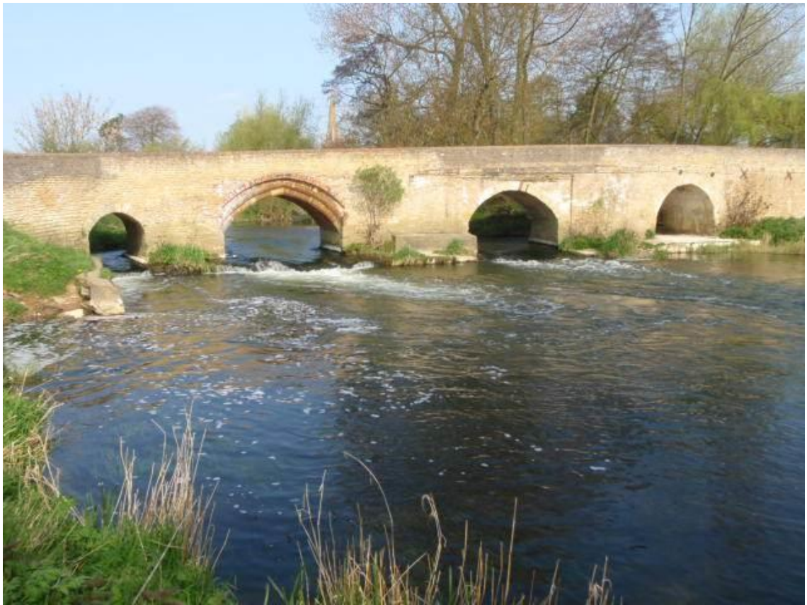
Figure 4.40. Harrold Bridge weirs at normal flow conditions, photograph taken from a downstream position.
